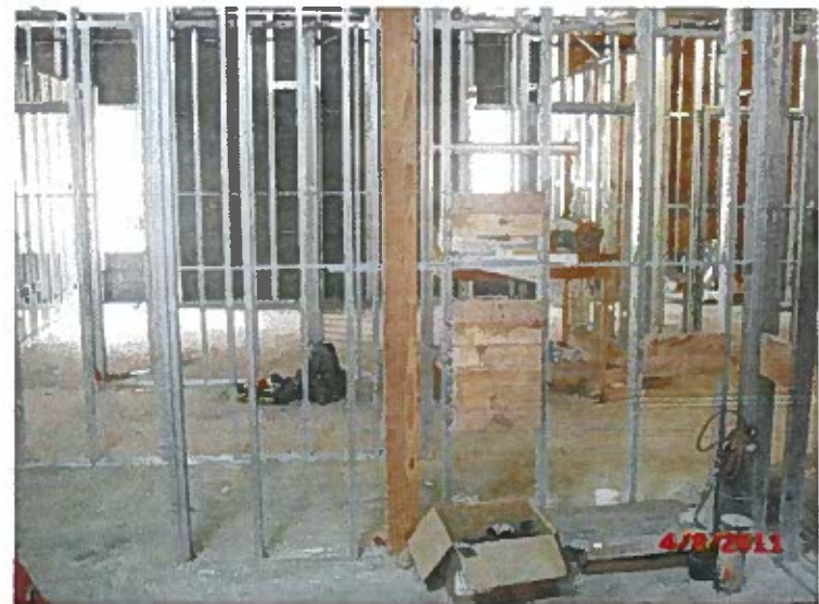
CSC Student Center - Grab bar and toilet partition blocking.
