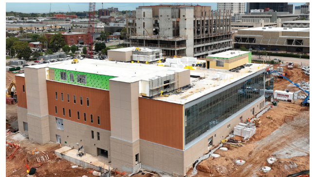
Construction continues on the new veterans hospital in downtown Tulsa, which will officially be named the James Mountain Inhofe VA Medical Center.
